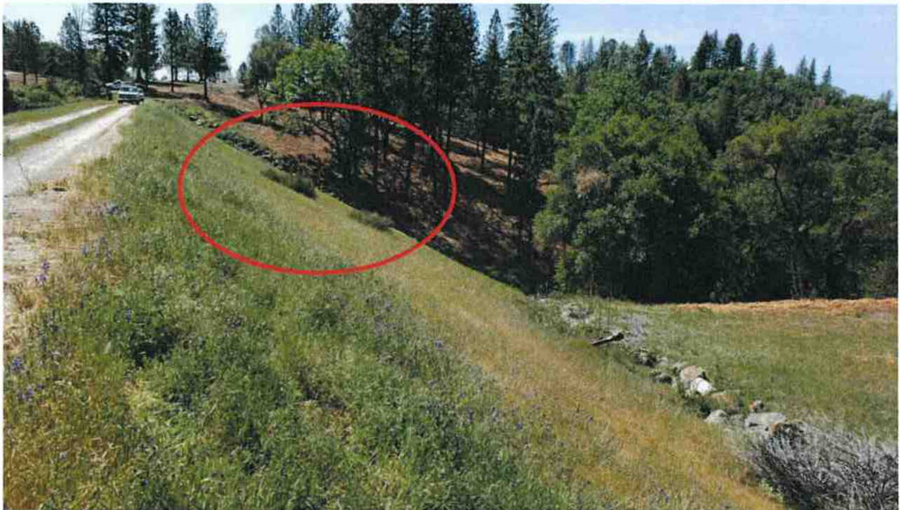
1. View of downstream face of the dam. Woody vegetation in red.
