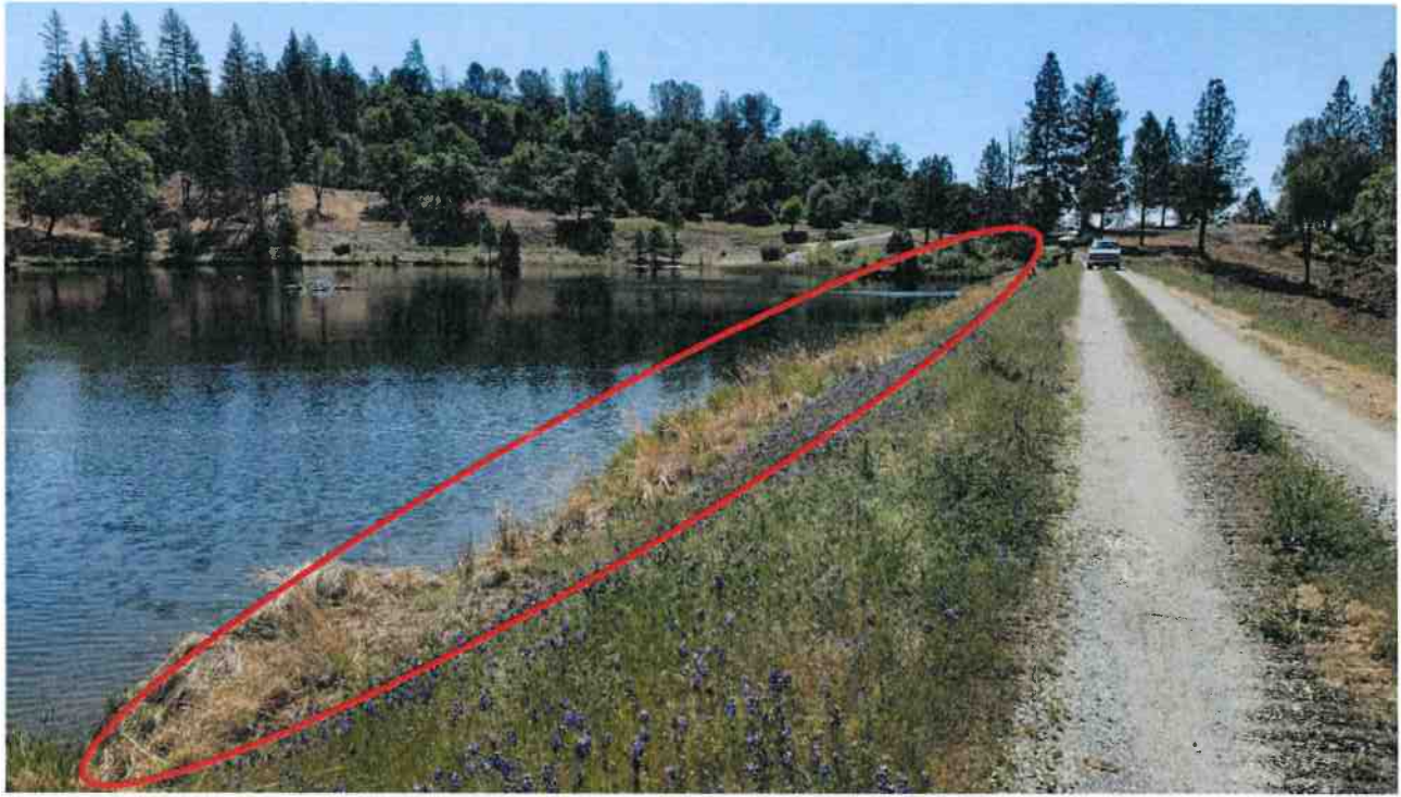
2. View of upstream face of the dam. Tules and vegetation in red.
